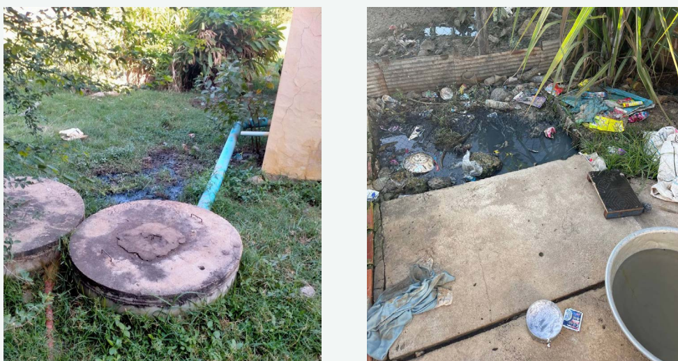
Figure 8. Evidence of overflow, surface ponding and uncontained excreta in Cambodia
