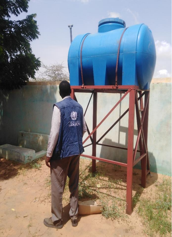
Figure 7: A water reservoir observed during the WASH assessment of one of the healthcare facilities in Sudan
