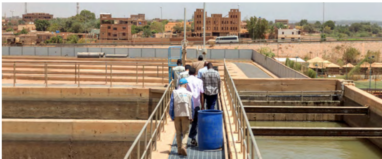
The UNICEF-supported plant provides safe water to more than one million people, Sudan. © UNICEF/UNI779677/Ahmed Mohamd
